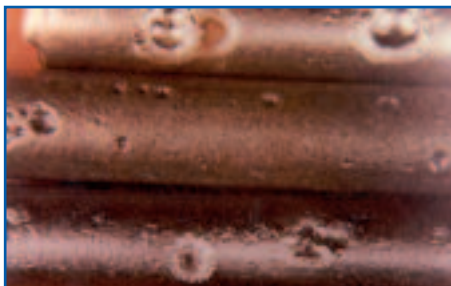
Figure 1 – Signs of hydrogen sulphide corrosion include shallow round pits with etched bottoms
